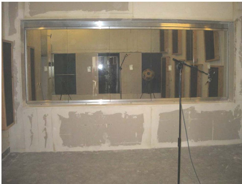
Fig. 1: View Transmission Room, Measurement 1
